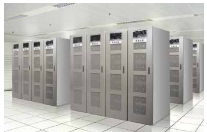
Backup power supply for livestock battery chamber
